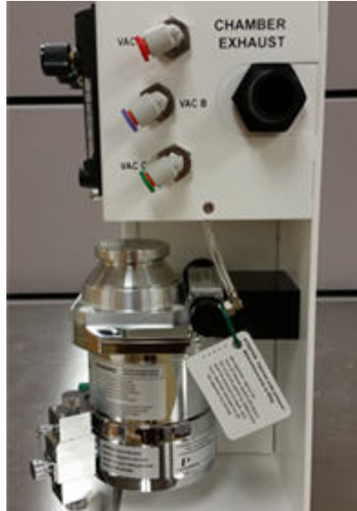
Figure 5. Vacuum and Chamber Exhaust Outputs
